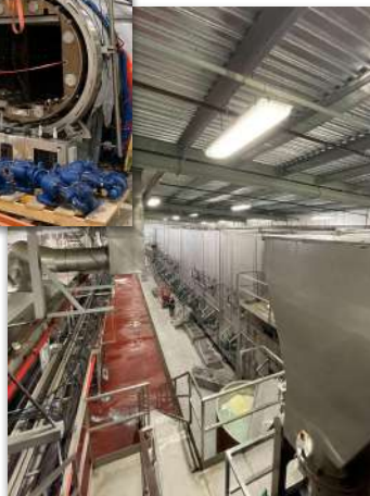
Tunnel de surgélation
